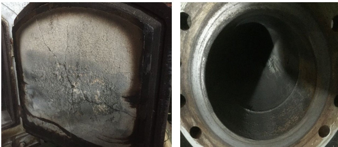
Gambar 2. Scale in Boiles and Pipe
