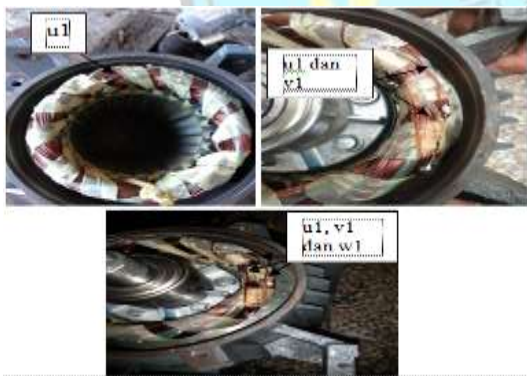
Gambar 3. Kerusakan Belitan Stator Turn To Turn
